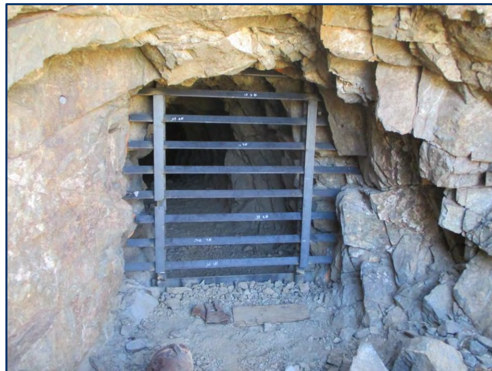
Grate that allows bats to move in and out of an abandoned mine adit in Arizona
