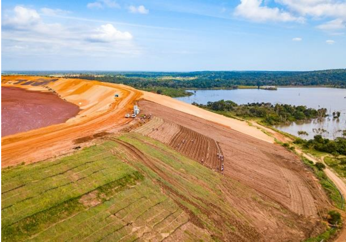
Base titanium tailings dam, 2017
